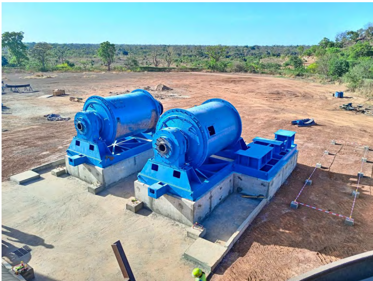
Figure 2 Ball Mills mounted on concrete footings
