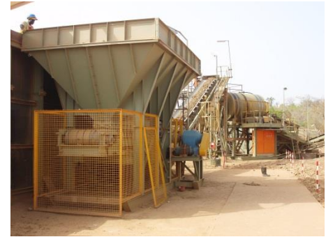
ROM BIN & FEED CONVEYOR
