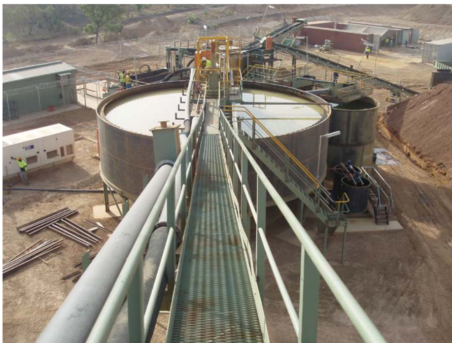
Figure 6 - View of gravity plant from 26 inch cyclone tower
