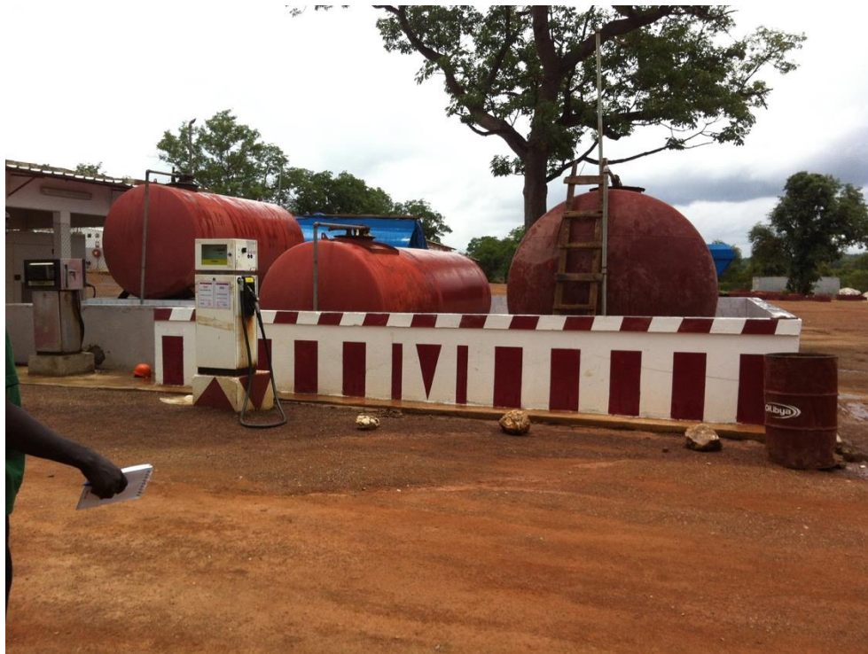
Figure 8: Douta Camp Diesel Fuel Facility – 85,000 Litre Capacity
