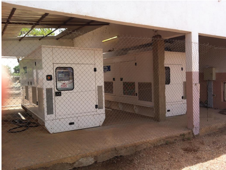
Figure 7: Douta Camp Diesel Genset Power Supply
