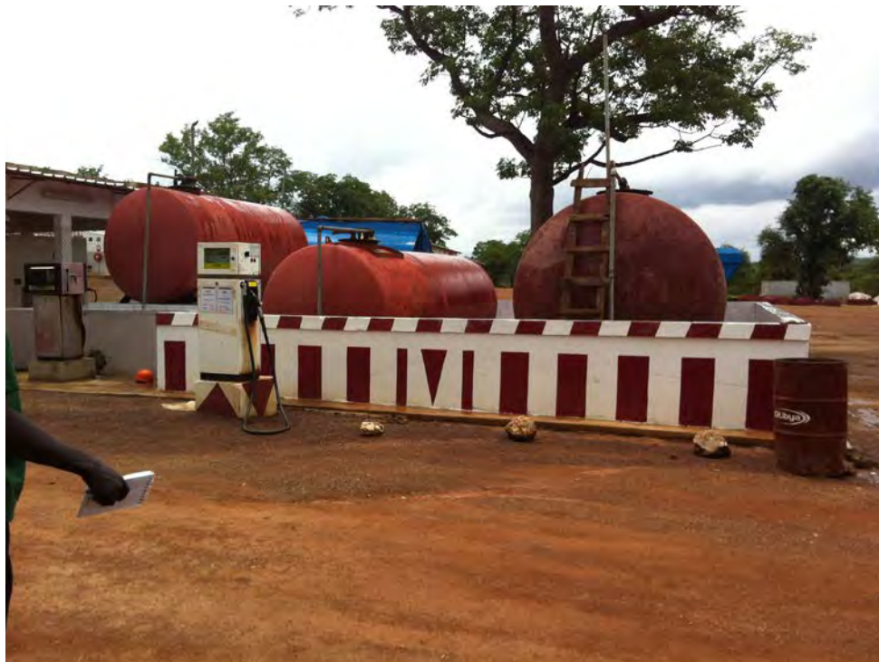
Figure 19 – shows the 85,000 litre diesel fuel farm within the Douta Camp.
