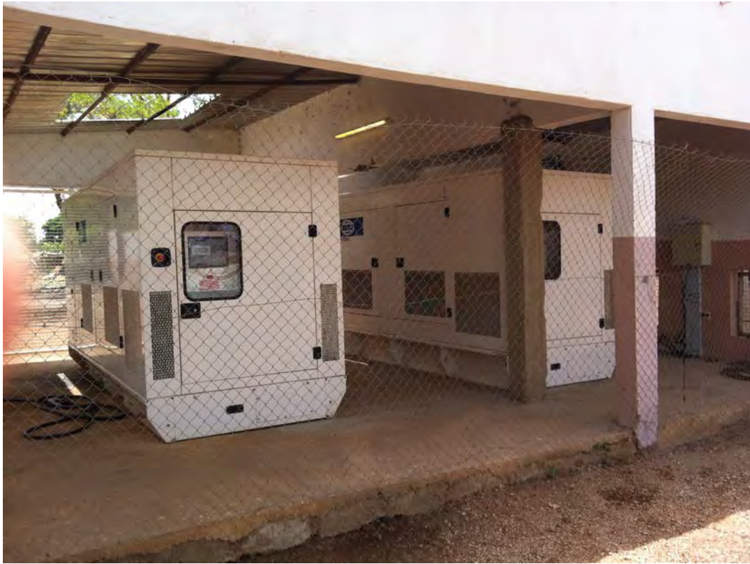
Figure 20 - shows the two Wilson 350kva gensets (1 duty, 1 standby) providing power to the Douta Camp.
