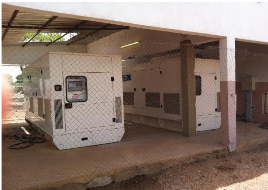
Figure 21 - shows the two Wilson 350kva gensets (1 duty, 1 standby) providing power to the Douta Camp.
