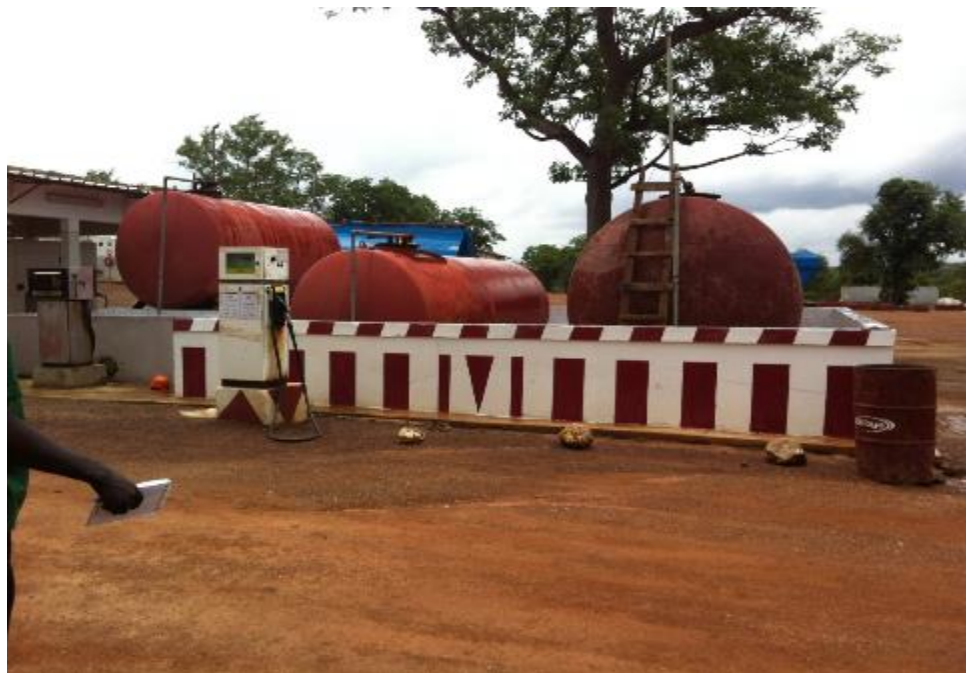
Figure 20 – shows the 85,000 litre diesel fuel farm within the Douta Camp.
