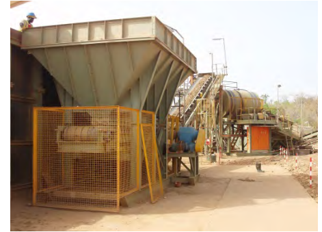
ROM BIN & FEED CONVEYOR
